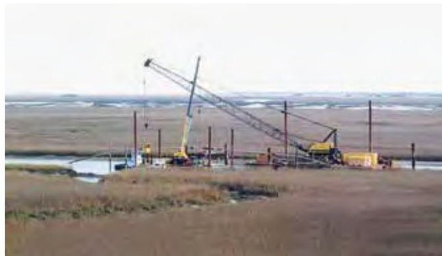
Figure 3 - HDD and cable splicing work platform within Hamlin Sound, SC situated in the marshland. The pipes carrying high voltage cables installed by HDD are being overboarded and buried below subsurface (Photograph courtesy of Pridmore and Varner/TD World.com)
