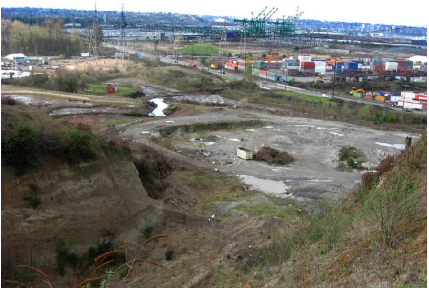
Site prior to construction. The project represents the Port of Tacoma's largest habitat restoration.
