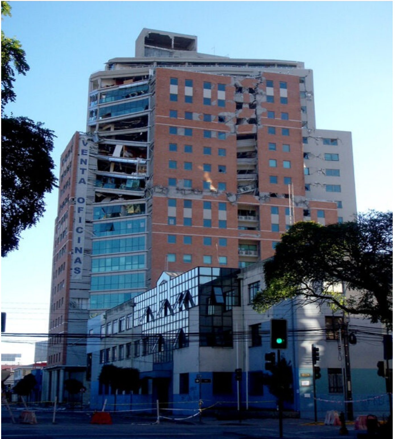
Earthquake-damaged new construction in Concepcion, Chile
